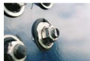
Exposed Nut/Washer combination prior to protective caps
